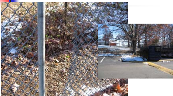
Fence Damage behind dumpster across from Bldg 44
